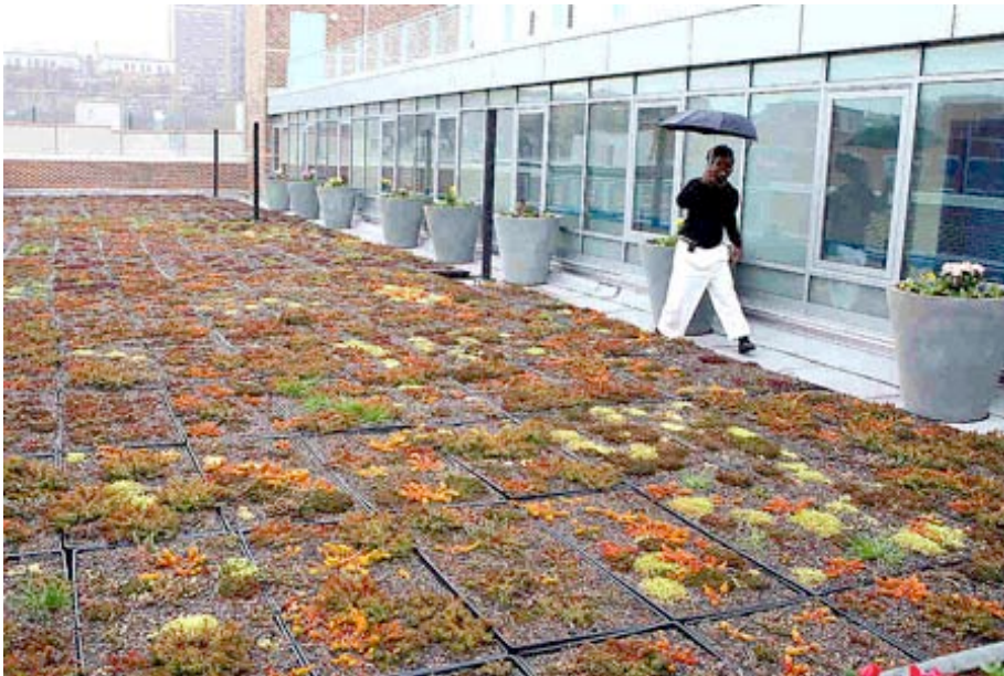
A green roof at David and Joyce Dinkins Gardens, a building offering affordable housing in Harlem.
